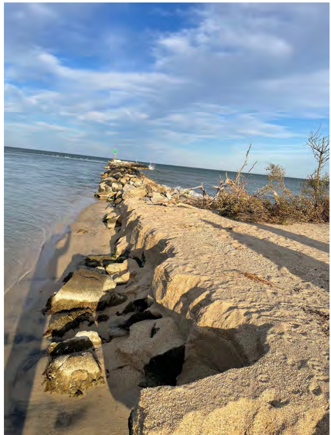
Figure 15. Reported conditions of the southern jetty after a storm. Photo taken Nov 5 th , 2025.
