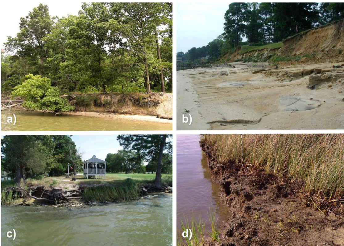
Fig 42. Sites with evidence of erosion.
