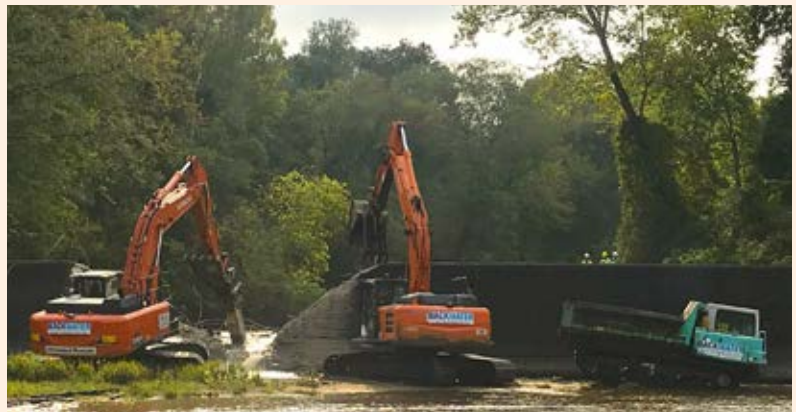
Heavy machinery works to demolish and remove the 1916 Ashland Mill Dam making way for migratory and resident fish species. Credit: Alan Weaver.
