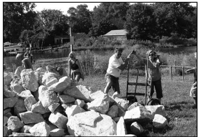
Figure 3. Contribution of volunteer labor: 200 volunteers contributed 800 hours to construction of the living shoreline in Glebe Bay, South River, Maryland.
