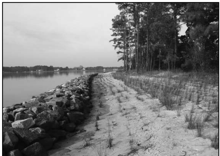
Figure 2. “Marsh sills” are used to contain sand fill that is planted with tidal marsh vegetation.
